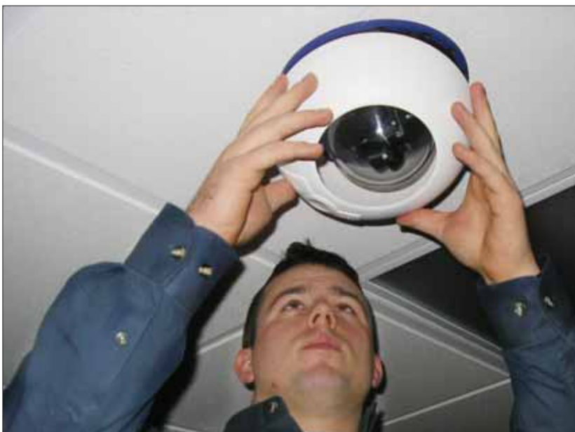
An alarm technician with ProTech Security Inc. of North Canton, Ohio, adds the finishing touches to an IP camera installed at Jackson High School in Stark County (Ohio).
